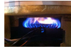
Storage Water Heater
